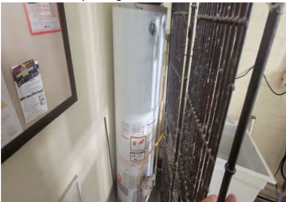
39 Building Water Heater
