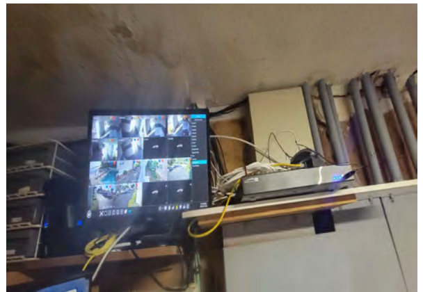
30 Building CCTV System
