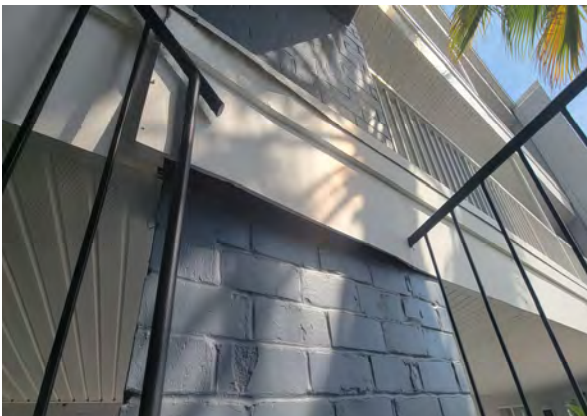
47 Loose Fascia Front Left Staircase
