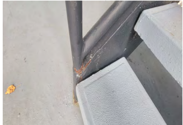
44 Deteriorated Weld at Front Left Staircase
