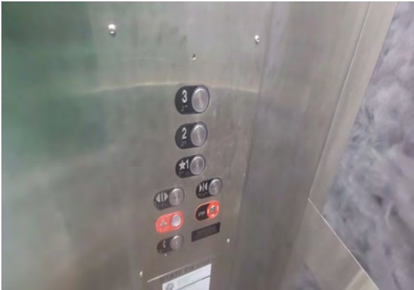
27 Elevator Floor Selection Panel
