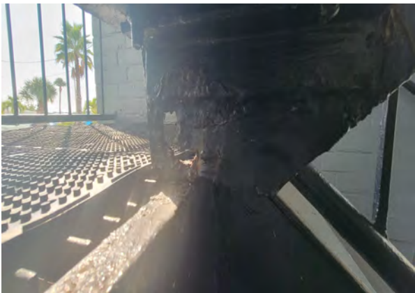
45 Deteriorated Weld at Front Left Staircase
