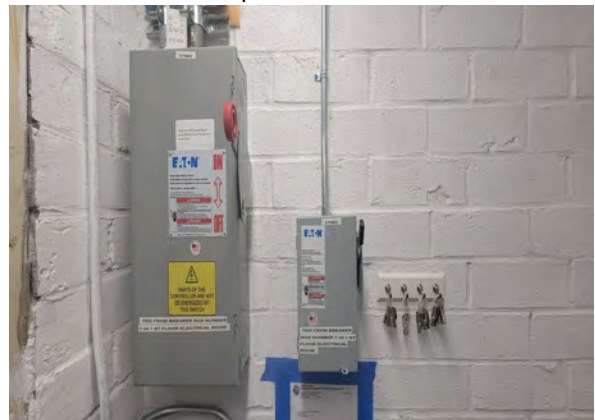
22 Elevator Electrical Disconnects
