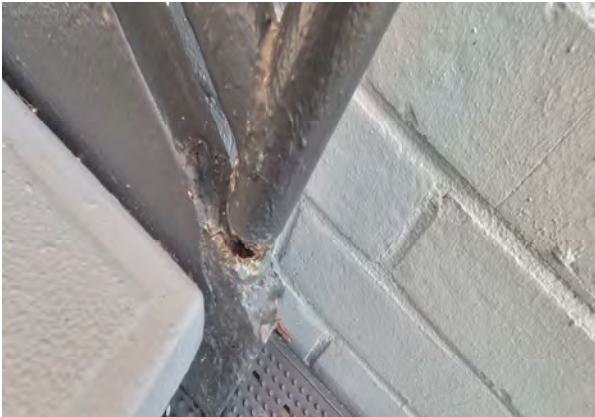
43 Deteriorated Weld at Front Left Staircase
